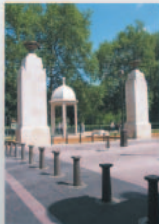
Access Control & Security - Hyde Park VP700 automatic bollard system
