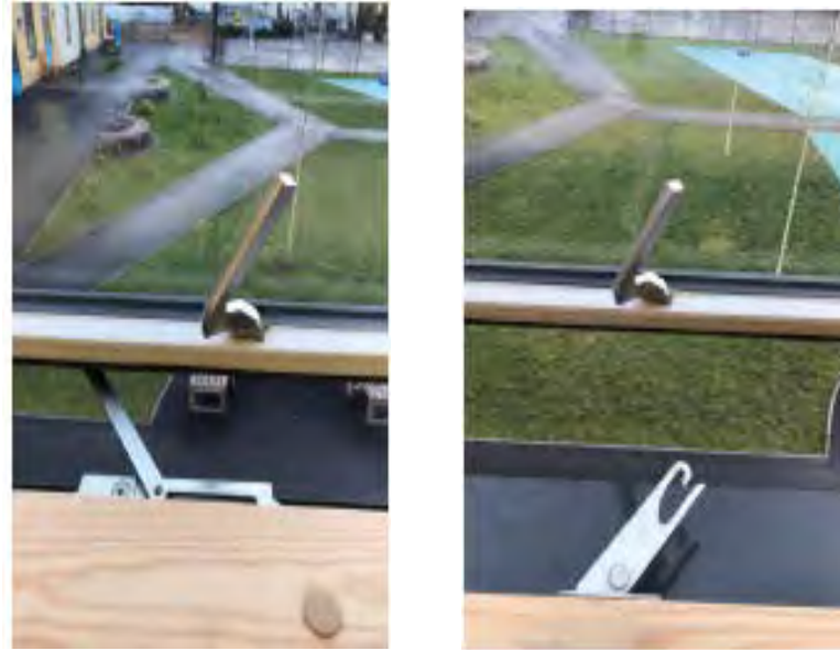
Problem window restrictor
