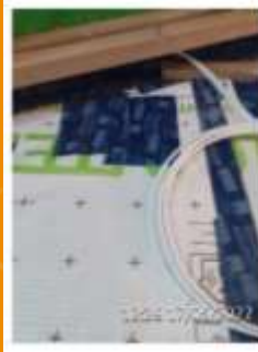
190 Assignee Lowfield Timber Frame Block A 1st floor - warmcell penetration
